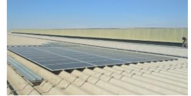
Pune plant, India (1MW)
