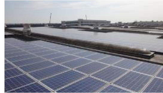
Wuxi plant, China (3MW)
