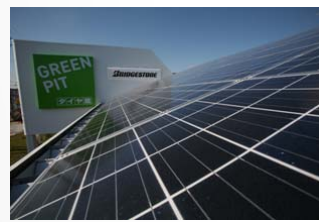
Solar modules installed as standard at “GREEN PIT” Tire Kan stores
