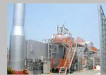
"Co-generation system" at Hofu Plant
