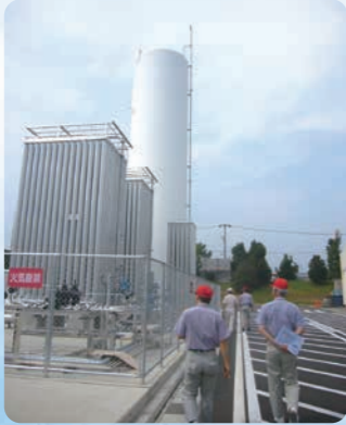
Natural gas tank in Bridgestone Iwata Plant
