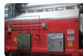
Introduced biomass boiler
