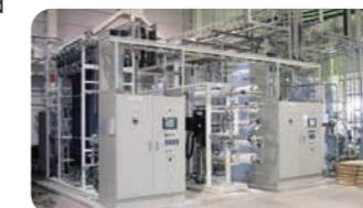
Water recycling system at Bridgestone's Kitakyushu Plant
